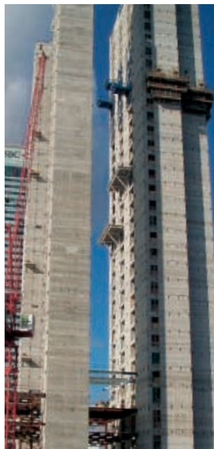
1 Installation of 24 units of the new Schindler 700 high-rise elevator in the One Churchill Place skyscraper, Canary Wharf, London, United Kingdom
